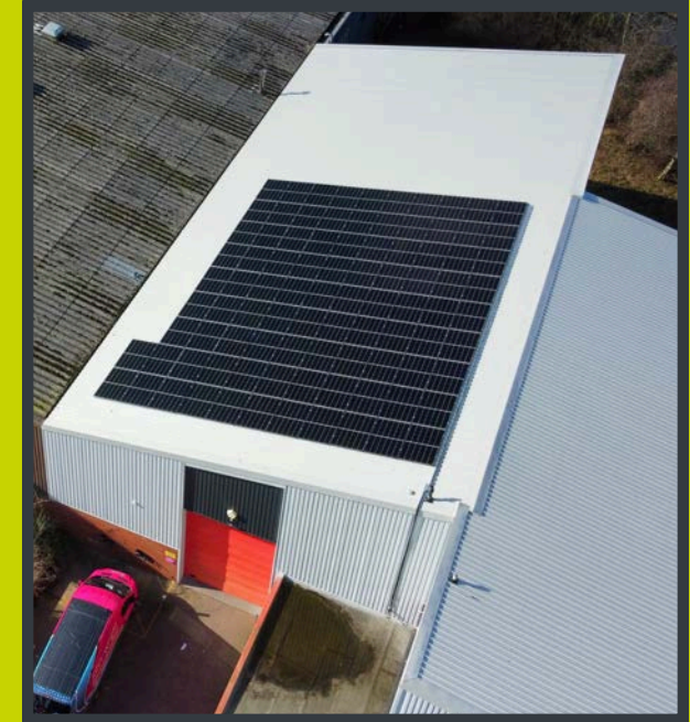
Solar panels at John E Wright
