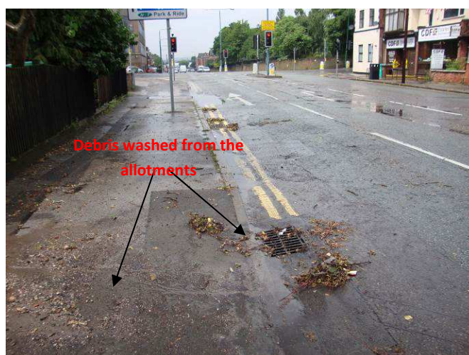
Figure 8: Flooding in 2012 on Haydn Road, east of Hucknall Road looking west towards the junction with Hucknall Road.
