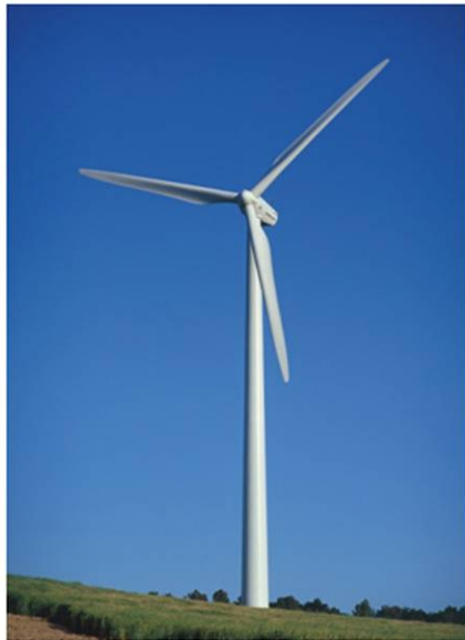
One commercial turbine (2.5 megawatt)
