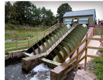
OR 4 hydropower plants (200 kilowatt)
