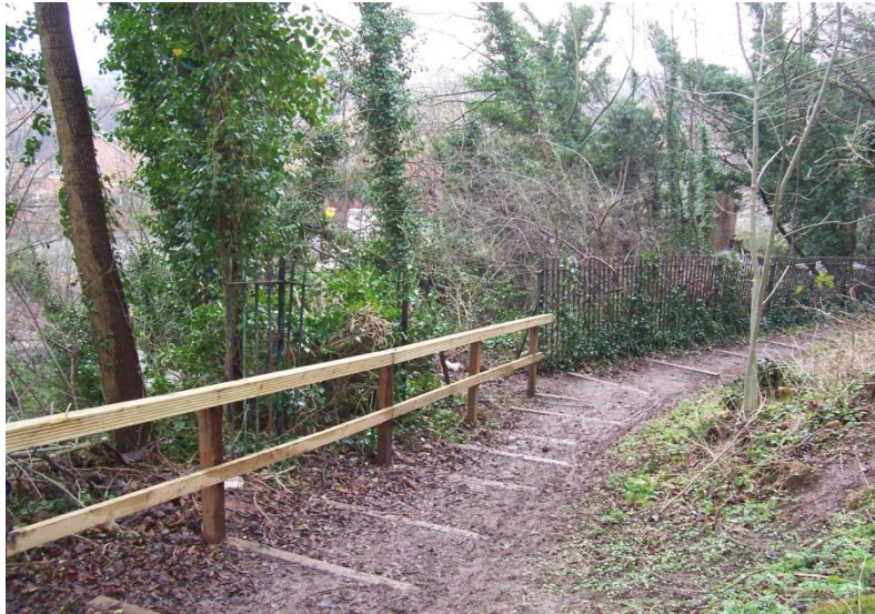
Figure 6: (after) handrail and sleeper steps have been installed along the steepest section. This has improved the overall accessibility of the path and reduced runoff and erosion
